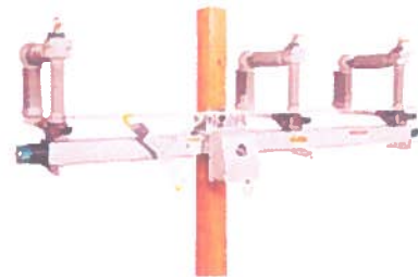
Figure 9. Overhead Loadbreak Switch
